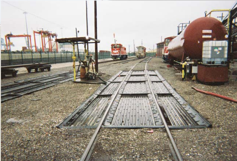
Pictured: Railroad Spill Collection Pans at Railroad Locomotive Fueling Station
