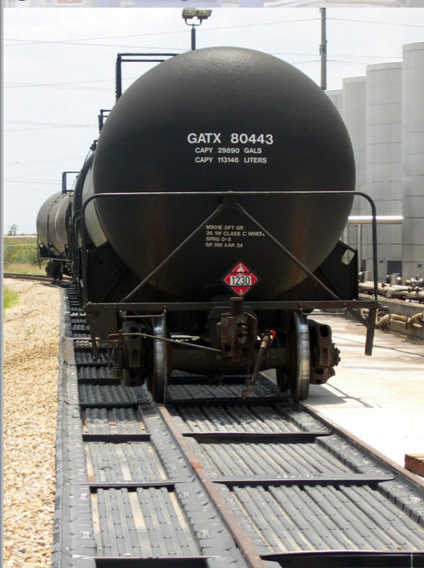
Century's Spill Containment System for Railroad Tank Car Loading Facility
