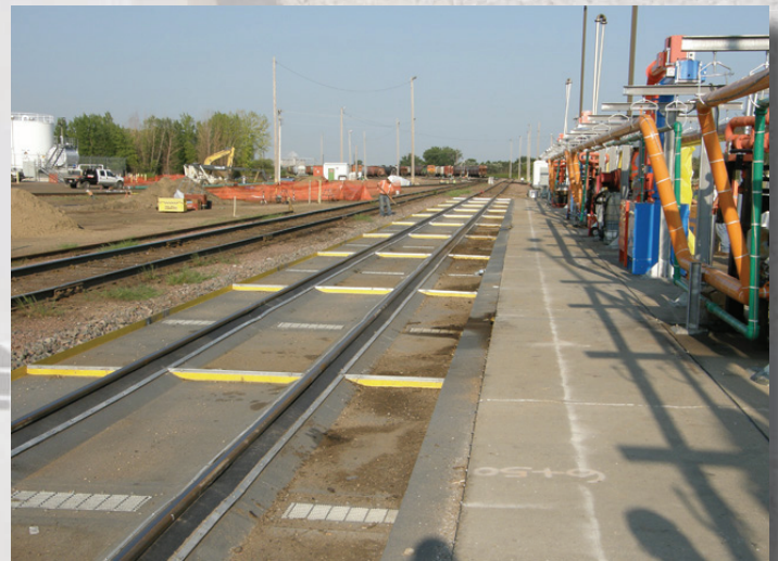
Galvanized metal railroad spill containment pans for a railroad locomotive fueling facility.
