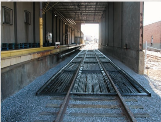
Railroad secondary containment food processing facility.
