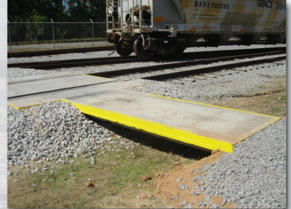
Century Group Inc's precast concrete pedestrian crosswalk installed in an industrial railroad spur.
