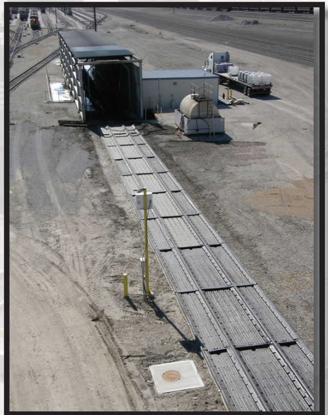
Century's HDPE spill containment system at railcar wash facility.
