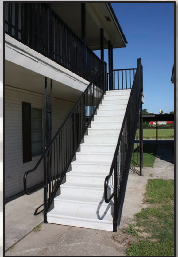
Closed Riser Stair Treads at Multi-Family Housing Project
