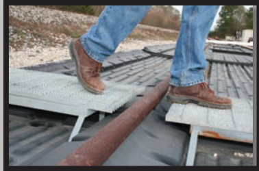
Elevated walkway on Century railroad spill containment pans.
