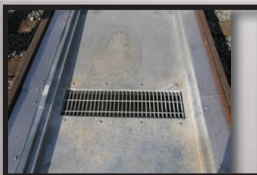
Recessed Grating Over Cross Drain
