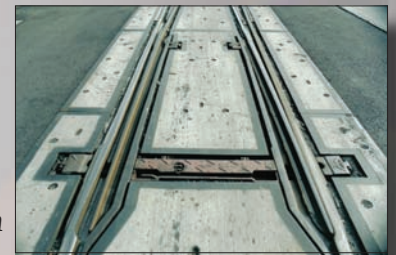
Custom Concrete Crossing In Tongued Switch
