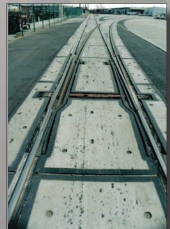
Custom Concrete Railroad Crossing In Turnout – Port Facility
