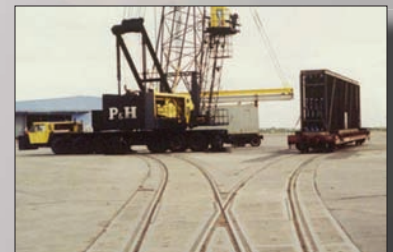
Turnout Concrete Crossing International Ports
